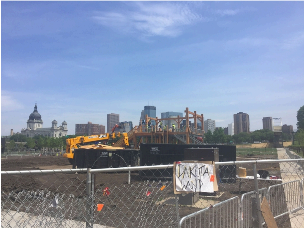
Dakota workers from Straight Line Construction dismantling Sam Durant’s “Scaffold” in the Minneapolis Sculpture Garden last weekend (photo by Sheila Regan/Hyperallergic)
